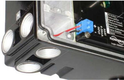
Figure 27: Conduit and Grounding
