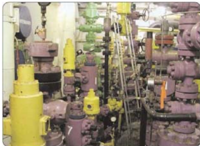
Space is precious in the Monopod well room Photo courtesy Flowserve Corp.
