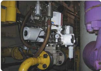
StarPac® intelligent control valve installed in the Monopod well room Photo courtesy Flowserve Corp.
