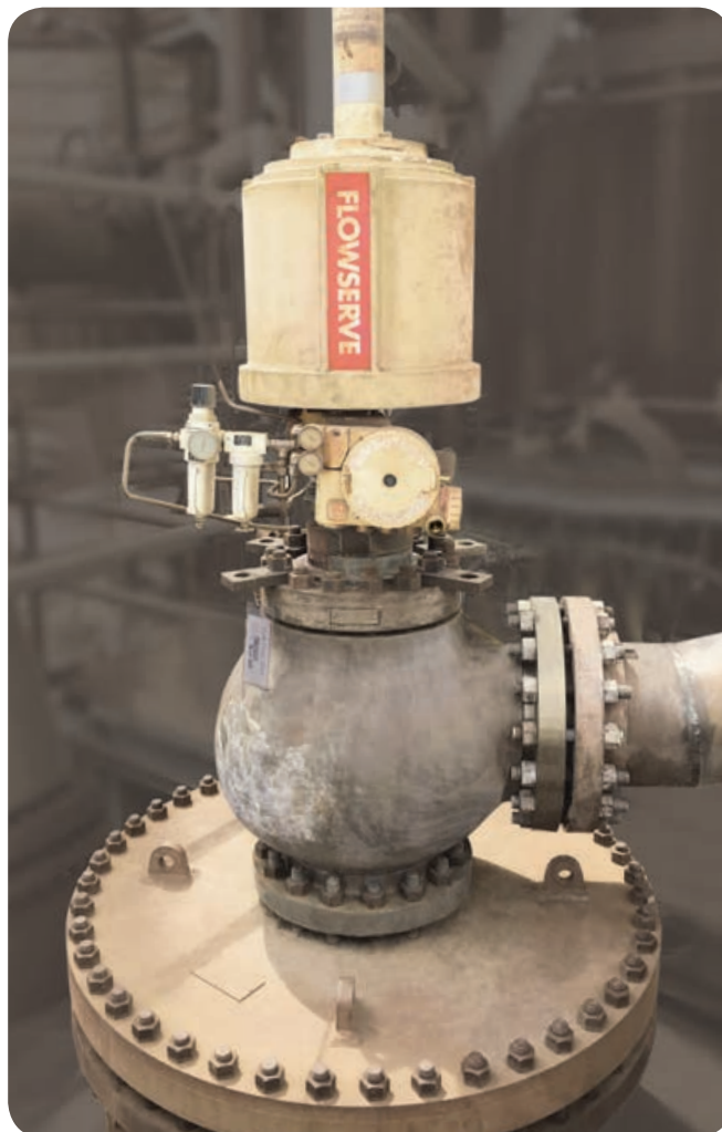
Valtek Survivor valve installed in flashing slurry letdown service
